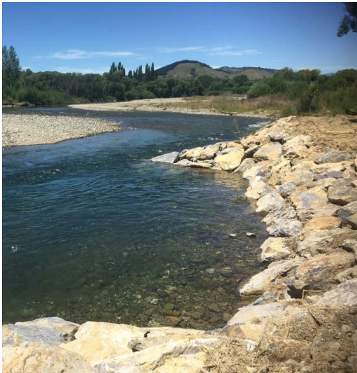
^ Rock groynes on the Upper Motueka. These provide better habitat for fish than rip rap.
