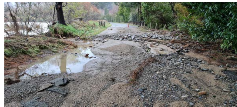
^ Damage to Westbank Road.
